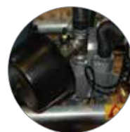
Blower inlet filter
